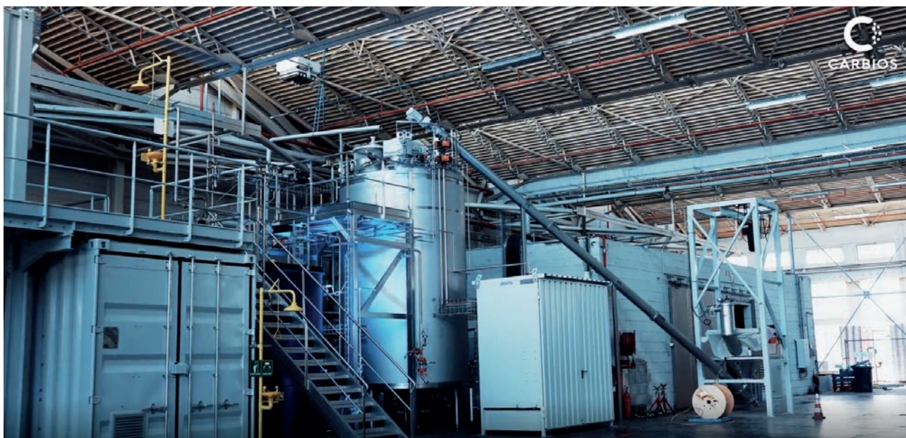
Carbios industrial demonstration plant for the depolymerization of PET plastic waste and textiles into monomers. (Carbios)
